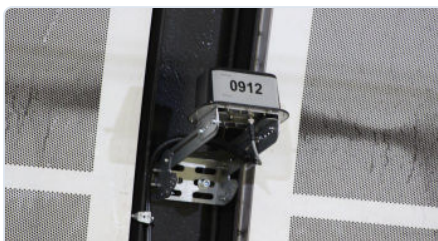
UWB Anchor — installed on wayside infrastructure like girders, or on tunnel walls using Piper's custom-developed bracketry.
